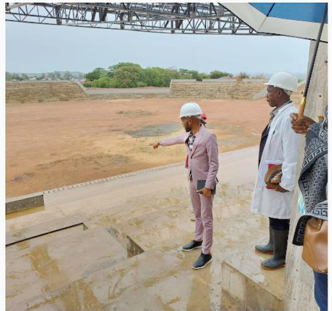
Director Amos Nyambo makes a point during the site visit at Mzimba Boma Stadium which at the time of monitoring was at 60%
